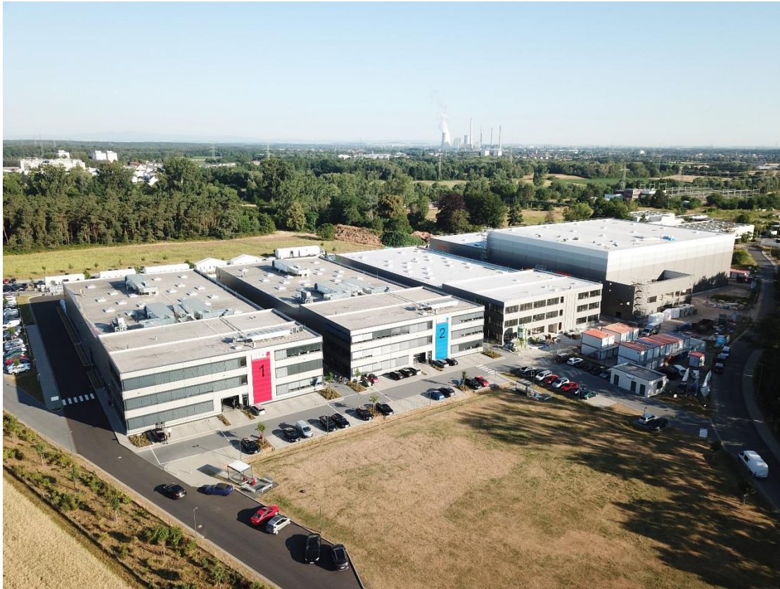
Caption: The headquarters of the BMZ Group in Karlstein am Main, where currently a third production hall and the logistics center are being built (1st and 2nd buildings from the right). In future, the battery systems for the JV will be produced in "Unit 3".
